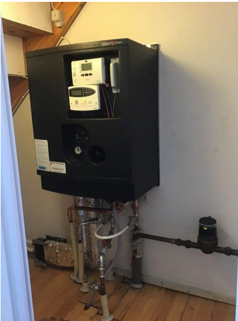
Figure 5. Final installation of a district heating unit (flat station) at a customer's dwelling in Østerby district
