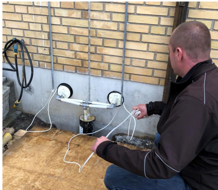
Figure 4. Connection of two dwellings to the service pipe of the district heating network in Østerby district
